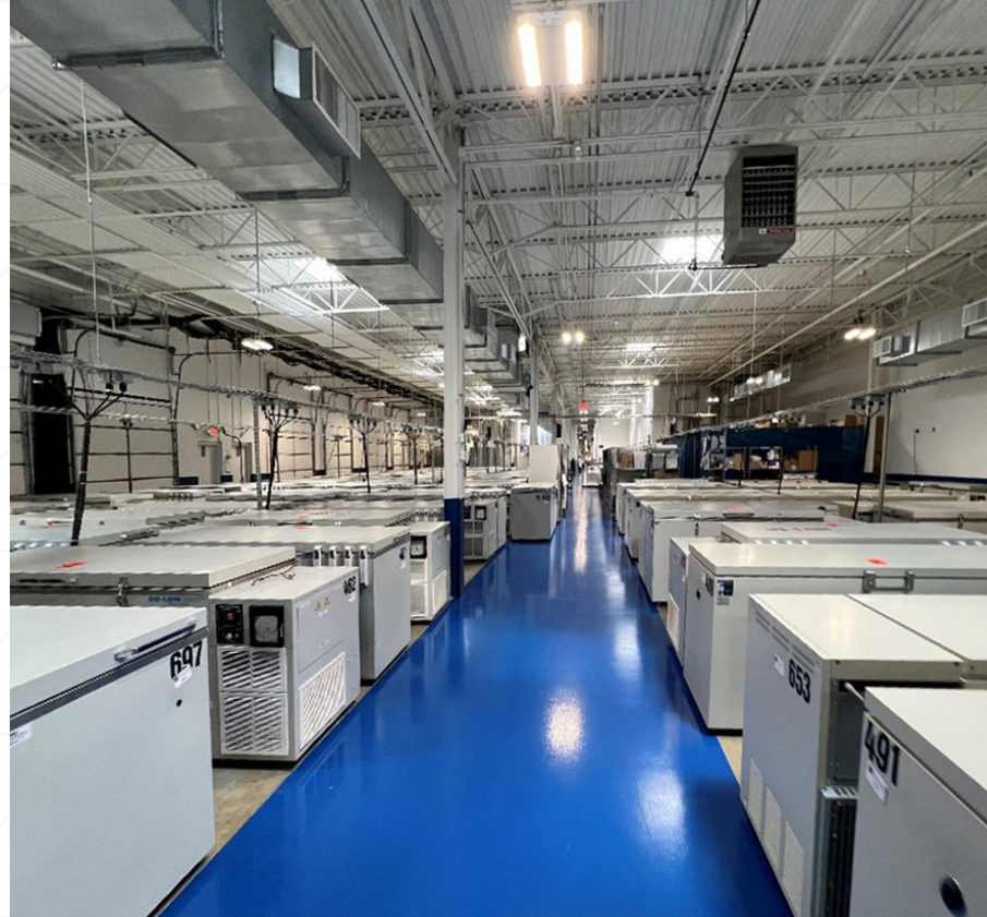
Installation of brighter, more energy efficient LED lighting in the biorepository of Precision's Frederick, MD laboratory will lower the facility's energy usage and associated GHG emissions.
